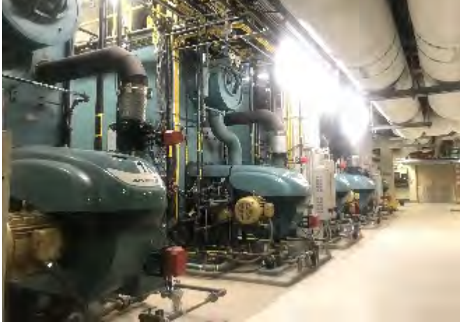
New Methodist Boilers
